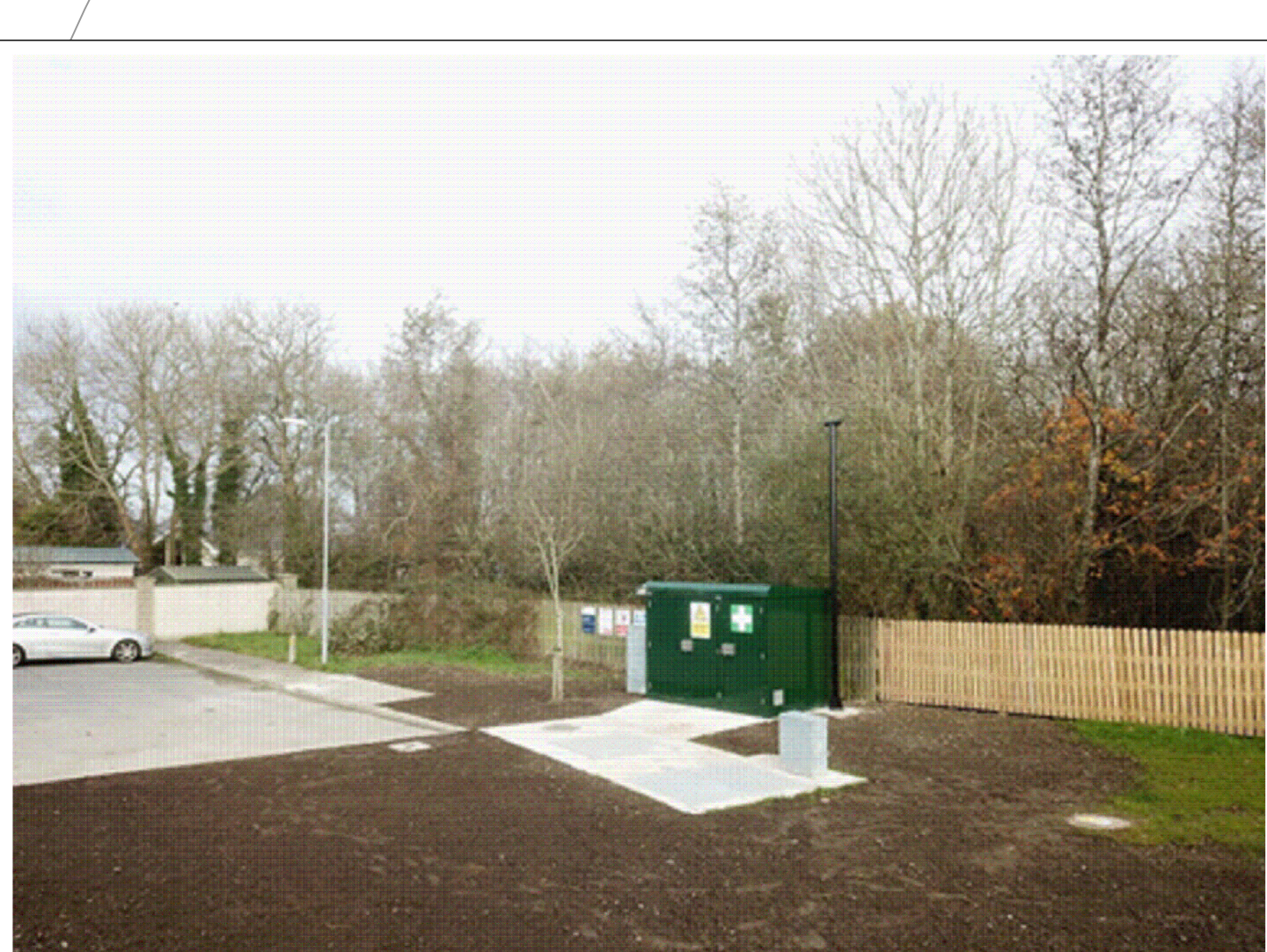
IMAGE 001 - FOUL PUMPING STATION EXAMPLE
